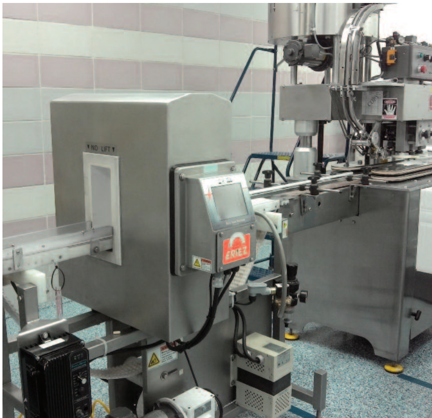
The DSP metal detector, shown here installed on a bottling line, uses the same interface as the other Eriez metal detectors at Global Health Industries. "If you know one, you know the other, and that just makes it easier for everyone," said Kim Wybrow, the company's production maintenance supervisor.
