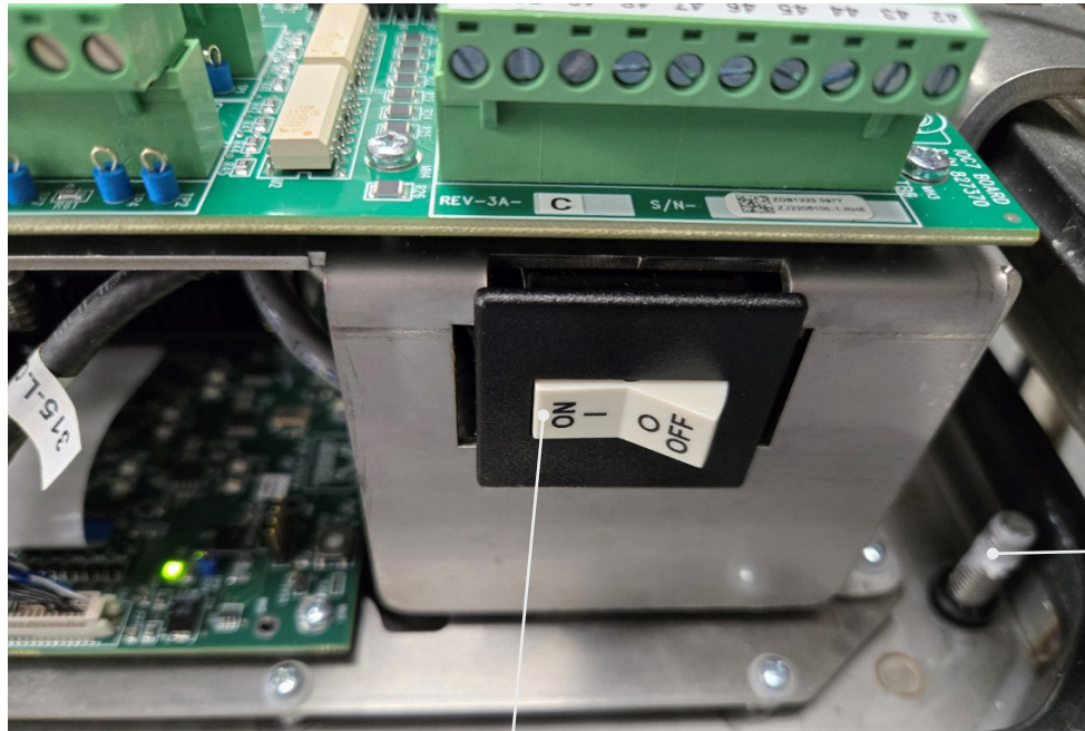
Main Power Switch 'ON' Position
