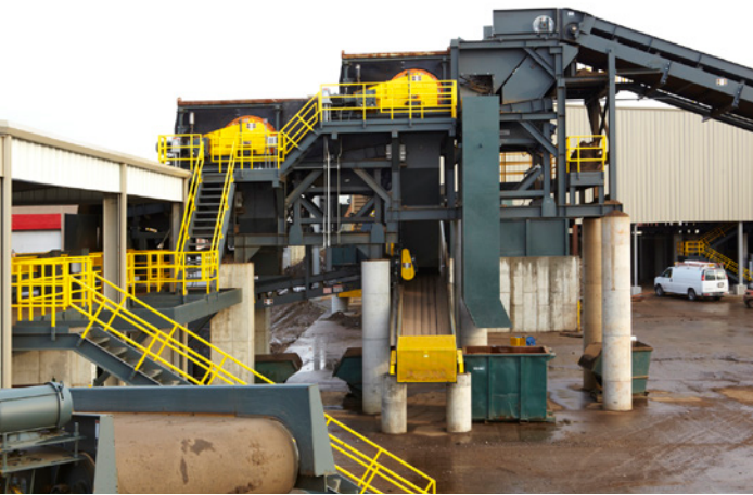
Garden Street's Spring Grove, Ohio, recycling operation incorporates advanced Eriez magnetic separation equipment.
